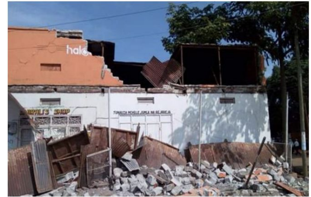
A collapsed building in Bukoba town, following the earthquake. Source: TRCS
